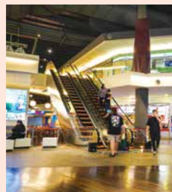
Replaced the North and South escalators connecting the Third Floor to the Third Floor Mezzanine
